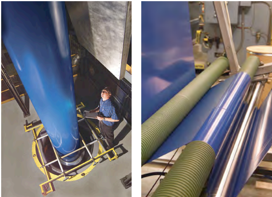
Vice-president of engineering Jim Antes (lower left photo) examines the film bubble on Argotec’s full-sized blown film line.
