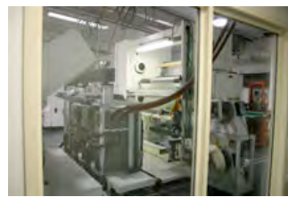
Argotec extrusion line in hard-walled cleanroom
