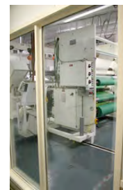
Argotec extrusion line in hard-walled cleanroom
