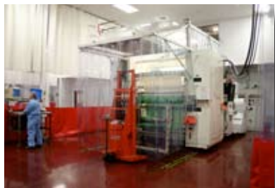
Multi-atmospheric hard-walled clean rooms
